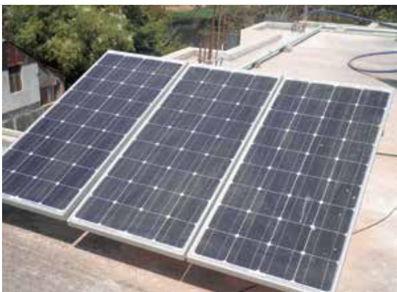
Solar panel of Rangamati Branch
